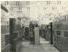
Fig. 7.—Interior view of the transmitting station.
